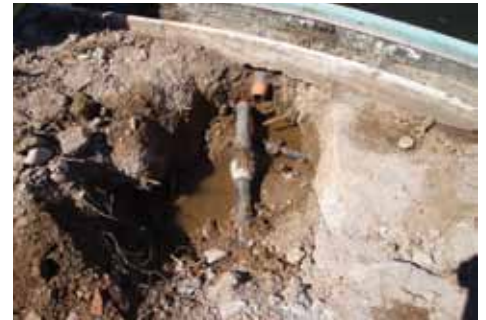
The repair workers were directed to open up the pavement where leaks were inspected, to find broken or cracked pipework, validating the results from the thermographic survey.
