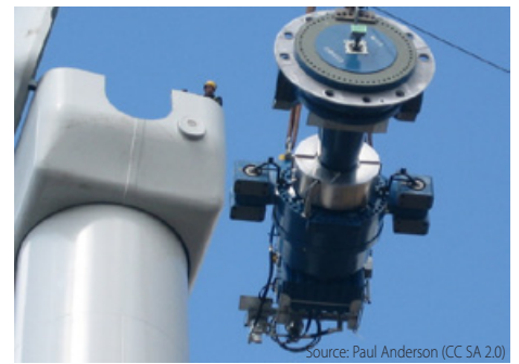
This huge 12 ton gearbox and disk brake assembly is lifted with a crane to a height of 60 meters to be mounted in this wind turbine nacelle.
