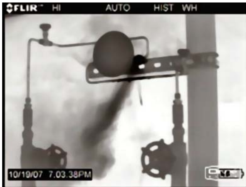
Figure 1. Propane leak imaged with FLIR GF320 hydrocarbon gas camera
